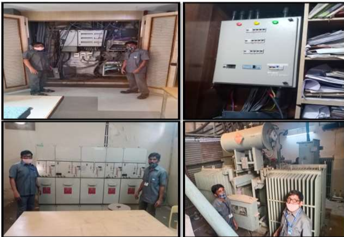
Walk-through Audit Conducted at various locations in UPG College Campus and the Energy Equipments were inspected
